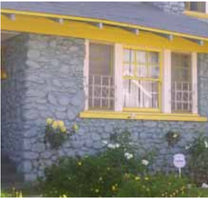
Stone and masonry should always be left to exhibit their natural finish qualities. Painting over the Arroyo stone on this house has muted the stone's texture.
