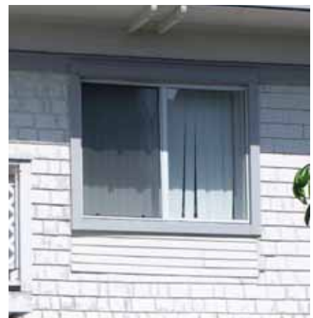
An inappropriately sized aluminum window diminishes the historic value of a house.
