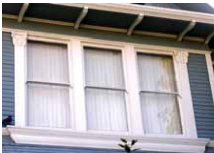
A window bay with decorative multi-light windows is shown at top. Grouped single-pane, double hung windows are shown below.
