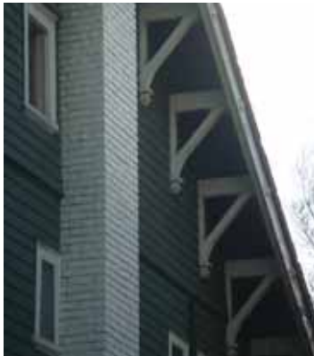
Details such as these decorative brackets are an important part of the roof.
