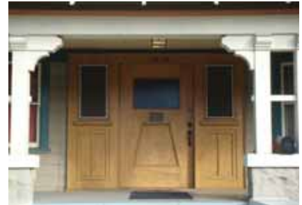
This door exhibits a natural wood finish, decorative panels, original hardware and side lights.
