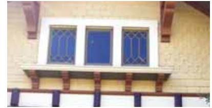
A tripartite attic window with fixed panes and decorative muntins is shown.
