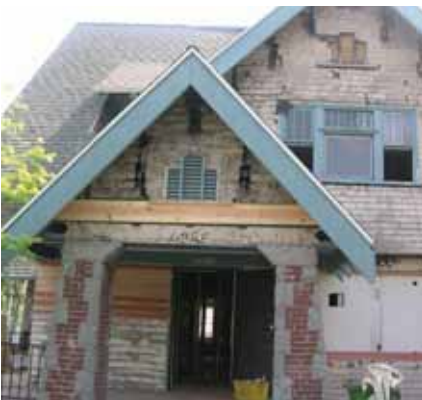
This house has recently been emancipated from a layer of stucco exposing ornate and beautiful materials.
